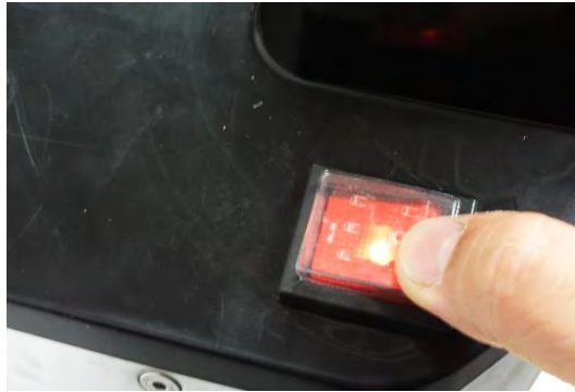
Picture 18: main switch
